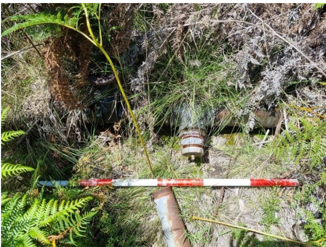
Photograph 21 Exposed pipe (D. Carpenter, 14 February 2024).
