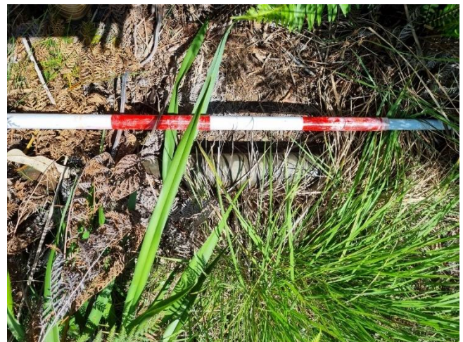
Photograph 22 Exposed pipe (D. Carpenter, 14 February 2024).
