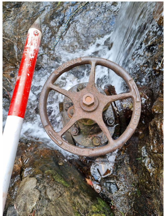
Photograph 18 Disused scour valve embedded in small weir to the west of Clover Dam Camps (North) (D.Carpenter, 14 February 2024).
