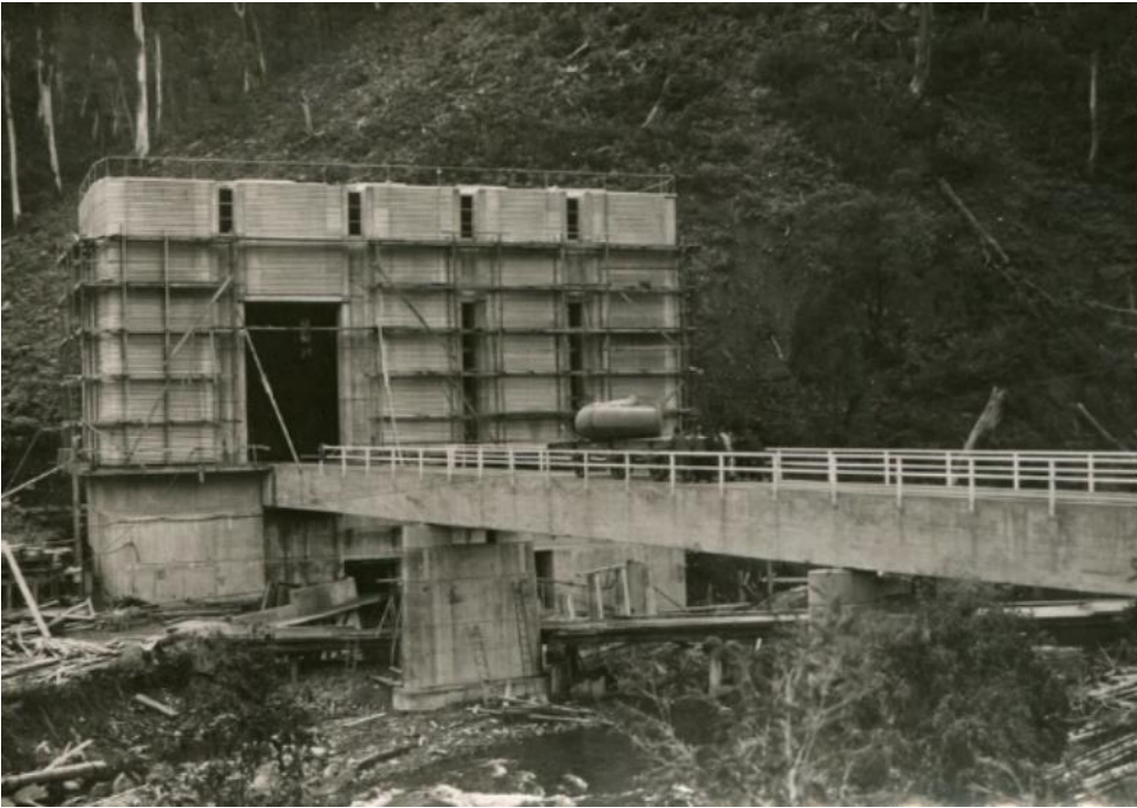
Figure 11 Clover Dam Power Station nearing completion, with the tail-bay location at the bottom of the photograph (Photographs - SECV - Clover Power Station, 1940s)
