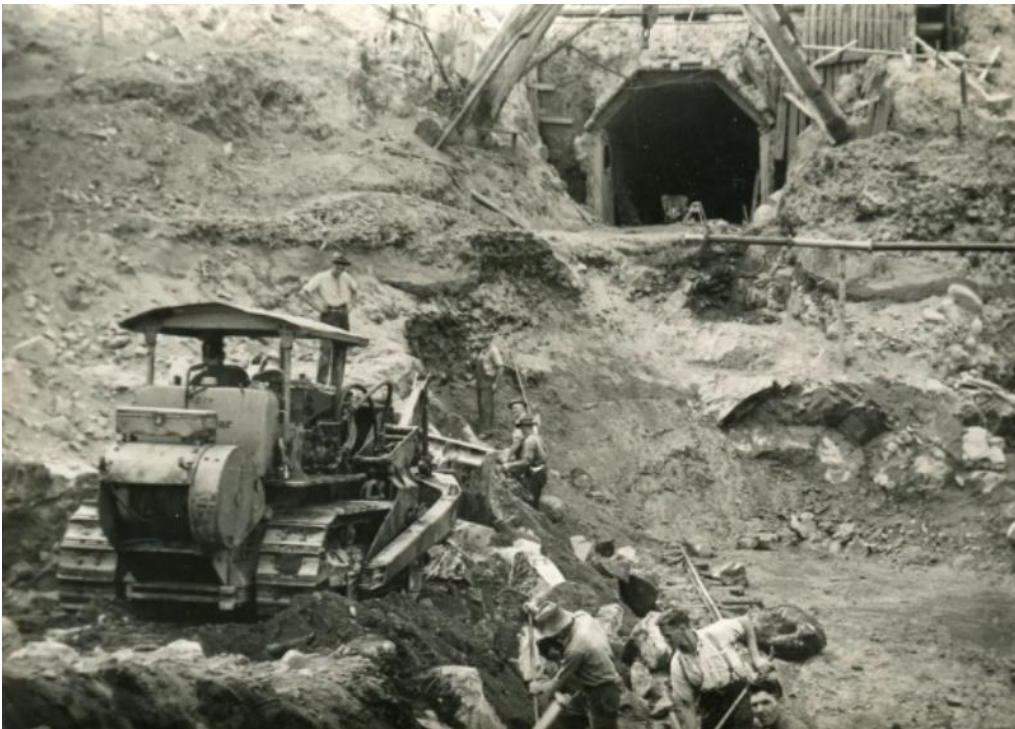
Figure 13 Image of combined manual and mechanical excavation occurring during the Kiewa Hydro Scheme construction (Photographs - SECV - Clover Power Station, 1940s)
