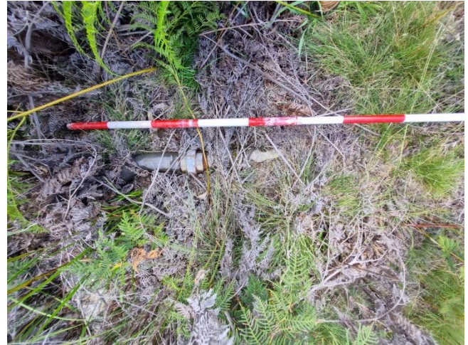
Photograph 20 Exposed pipe (D. Carpenter, 14 February 2024).
