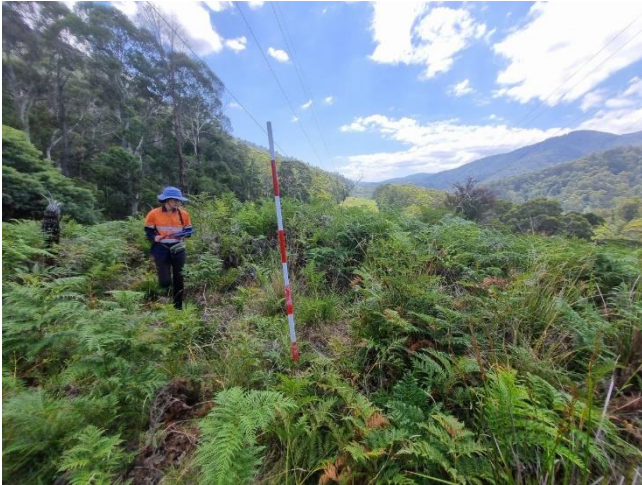
Photograph 19 Context of location of exposed pipe (facing north, D. Carpenter, 14 February 2024).
