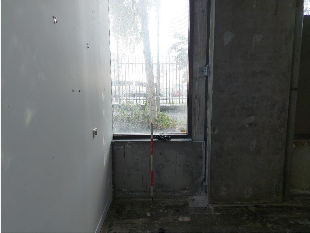
Figure 6: Demonstrating interior floor surface, towards centre of building, is significantly lower than exterior (see Figure 6), view south
