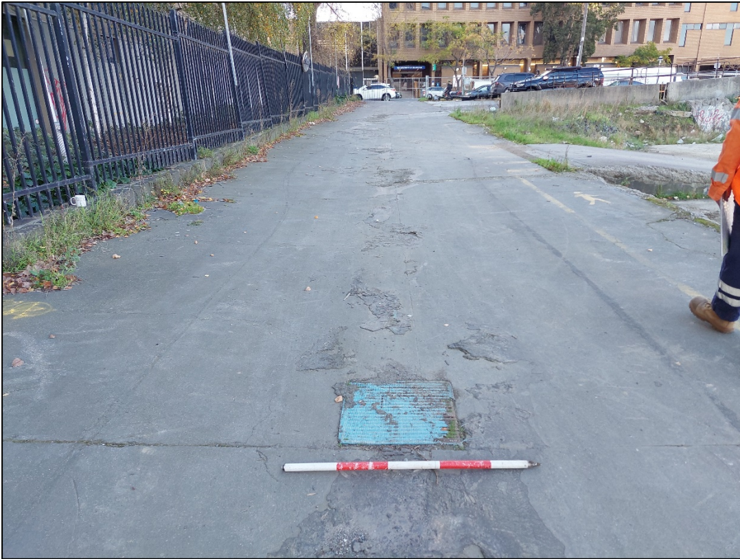
Figure 8: Drainage grate on the naturally sloping access road, view south-east (A. Valka, 26/06/2024)
