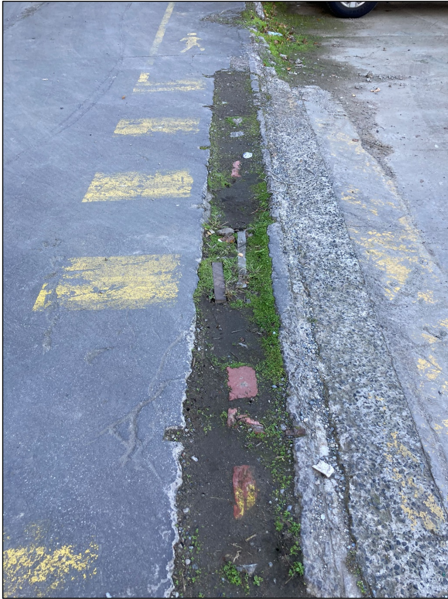
Figure 10: Row of bricks in between the concrete access road and 1980s cut, view north-east (R. Hocking, 26/06/2024)
