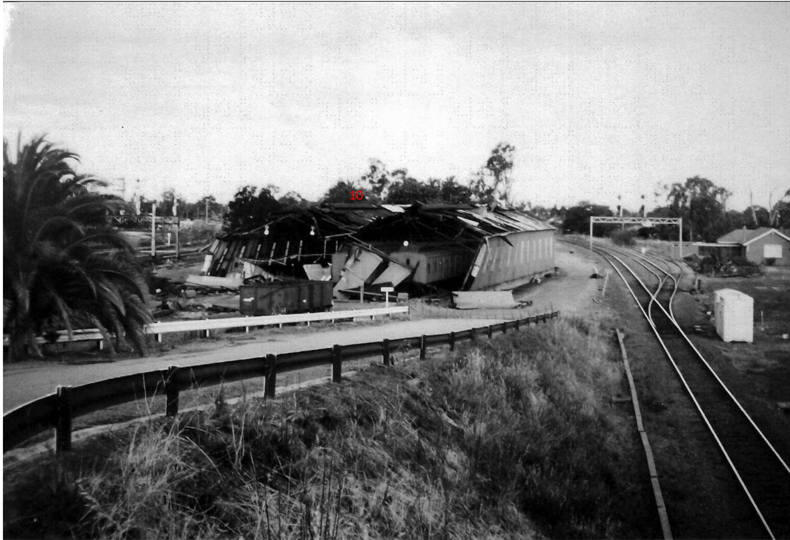
Plate Error! No text of specified style in document..16 Locomotive workshop in 1994 following collapse during storm
