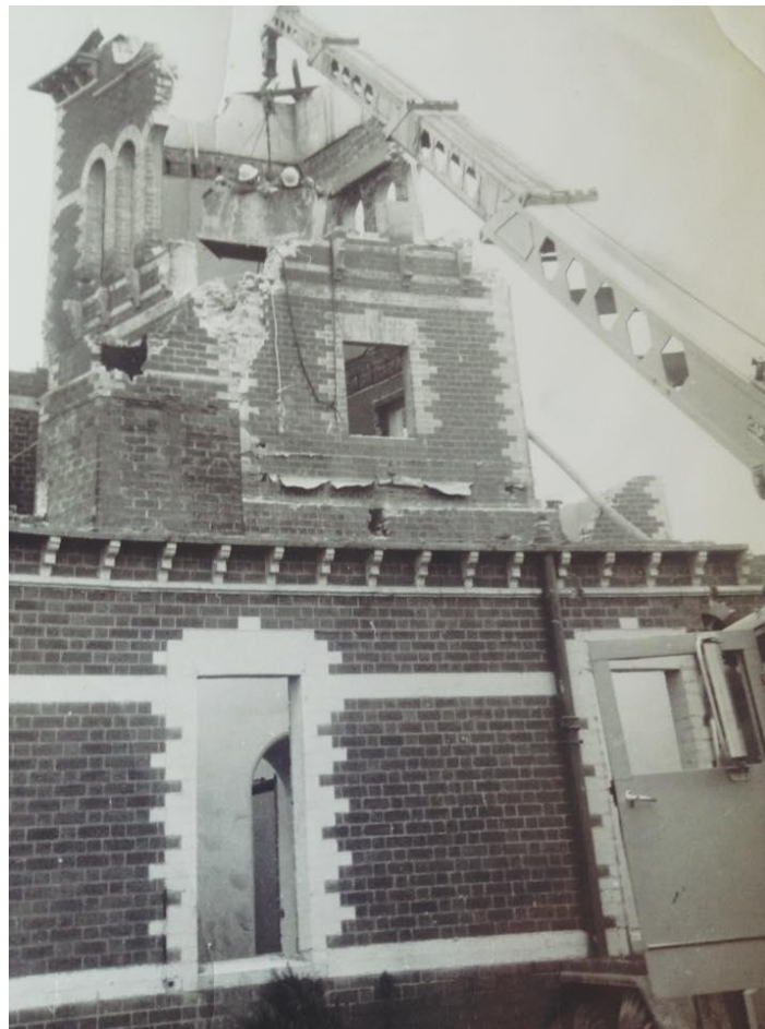
Plate 3.3 Demolition of the clock tower at Benalla Railway Station, November 1974 (Source: Benalla Railway Project Inc. https://www.facebook.com/978316085601467/ )
