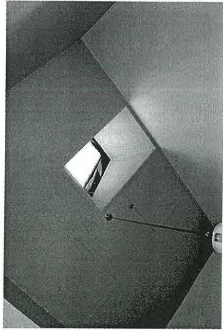
Photo 3.44: Interior, Office (spaces FF01-02). Detail of introduced strapped ceiling and original (altered) skylight.
