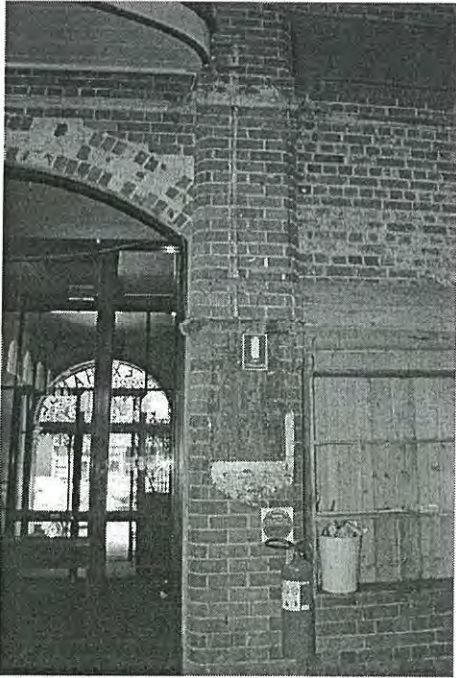
Photo 3.69: Interior, Exchange Hall (space H01). Detail of altered central archway on west wall.
