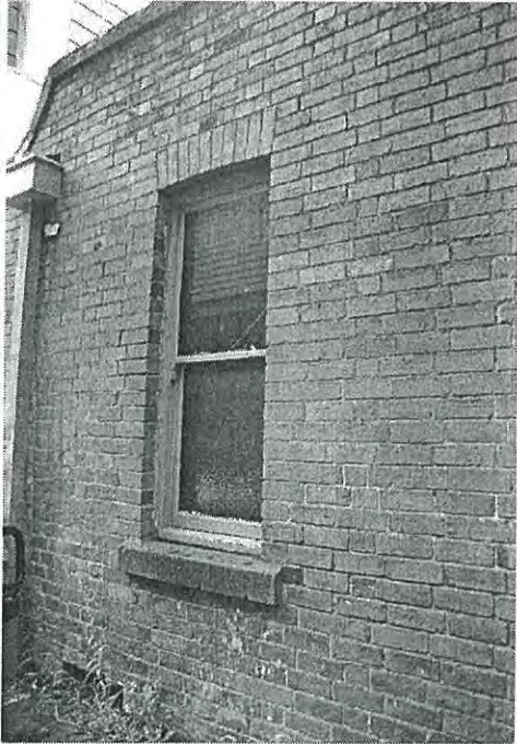
Photo 3.23: Exterior, Office & Toilet Wing, part west elevation (north end) showing early timber framed double hung window with early bluestone sill.
