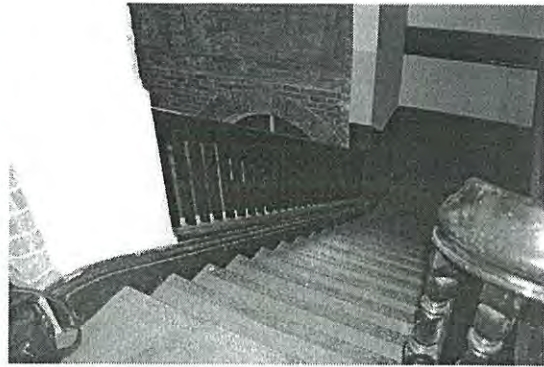
Photo 3.38: Interior, Landing & Stairs (space FF12). View of upper flight of stairs. Note the introduced timber stair balustrade (to the left).
