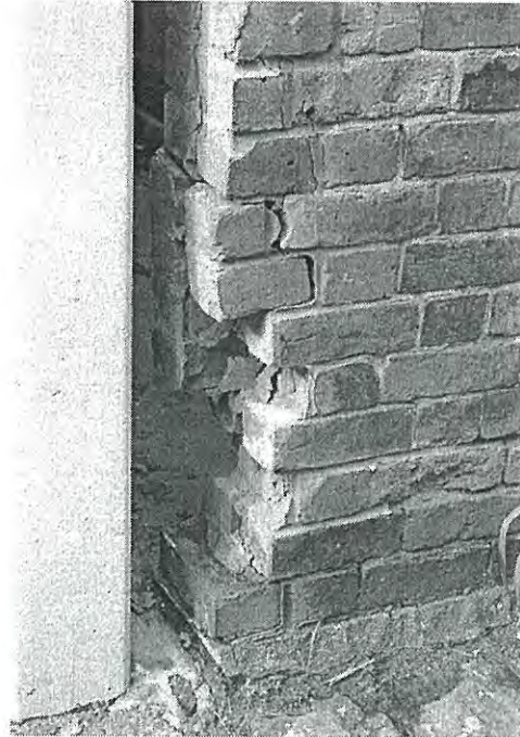
Photo 3.24: Exterior, Office & Toilet Wing, detail of damaged/partially demolished north-west corner of west elevation.
