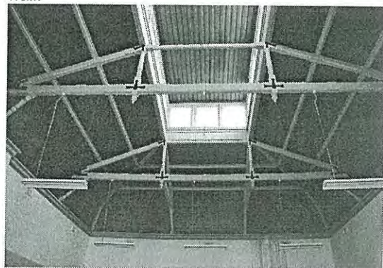
Photo 3.86: Interior, Call Room (space CR01). Detail of coved ceiling, Queen Post trusses and lantern light, looking east. Note the evidence of falling damp on the east wall, south end.
