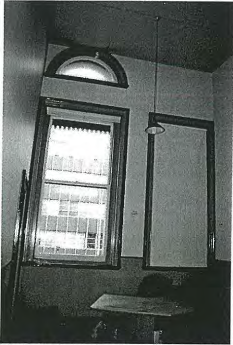
Photo 3.53: Interior, Office (space FF06). View of west wall showing timber framed double hung windows and semi-circular window.
