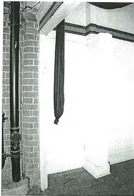
Photo 3.78: Interior, Booth (space B01). Detail of projecting wall nib, and blocked up door opening (west wall).
