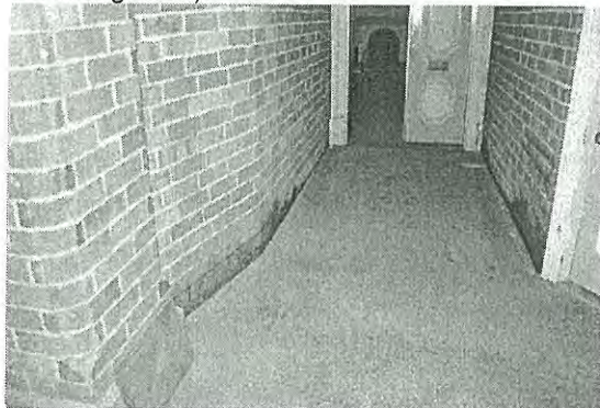
Photo 3.79: Interior, Exchange Hall (space H01). Detail of northern passage to call room showing evidence of rising damp on the lower courses of the brick walls.
