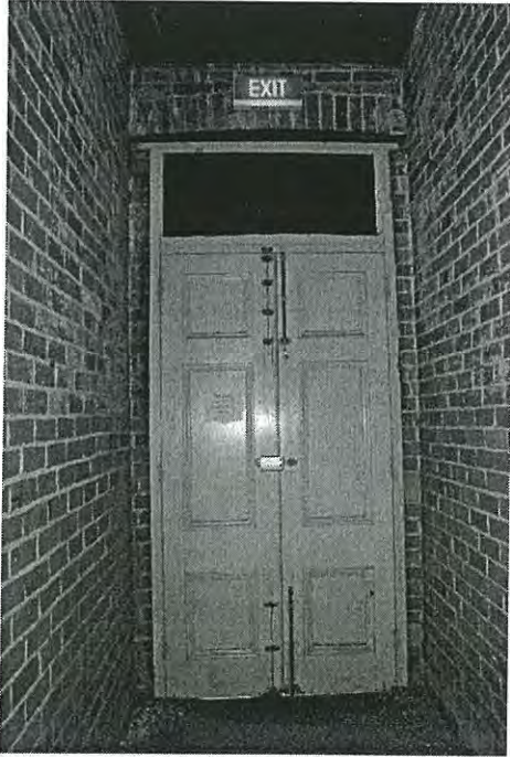
Photo 3.81: Interior, Exchange Hall (space H01). Detail of panelled timber double doors in rear passage forming eastern exit. Note the introduced door frame (especially evidence above the timber framing of the transom window which does not follow the curve of the original shallow arch).
