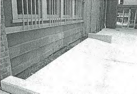
Photo 3.15: Exterior, Exchange Hall, detail of ramped concrete ground level adjacent to the introduced windows and wall cladding on the east elevation. Also note the space between the introduced concrete ramp and the wall base.
