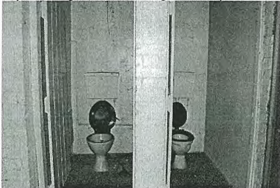
Photo 3.97: Interior, Men's Toilets (space T01). Detail of remaining toilet cubicles. The third cubicle (which was situated to the right of the photo) has been demolished.
