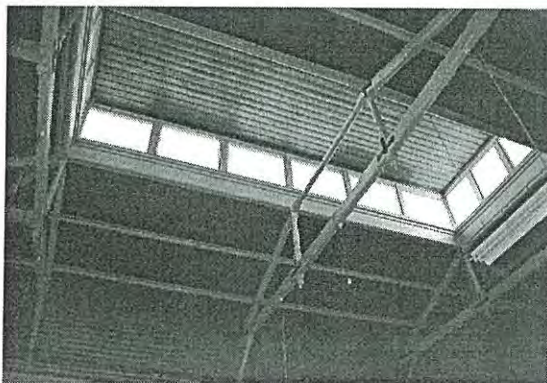
Photo 3.85: Interior, Call Room (space CR01). Detail of lantern light and Queen Post trusses.
