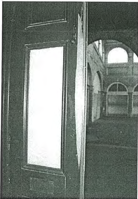
Photo 3.89: Interior, Call Room (space CR01). Detail of damaged door, showing fractured timber edge.
