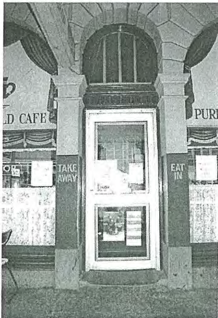
Photo 3.05: Exterior, Front Pavilion, detail of introduced aluminium framed and glazed door on ground floor shopfront, west façade.
