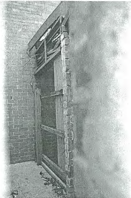
Photo 3.25: Exterior, Office & Toilet Wing, detail of open space showing partial demolition of toilet cubicle, timber framed galvanised corrugated iron partition (north end) and introduced raised concrete slab.
