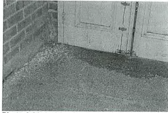
Photo 3.82: Interior, Exchange Hall (space H01). Detail of dampness under door opening and evidence of rising damp on the lower courses of the northern brickwork. The powdery nature of the mortar has left a residue on the floor.
