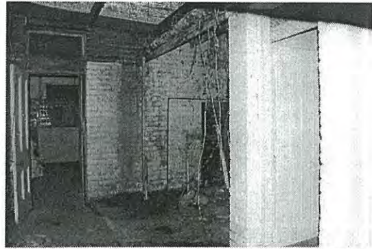
Photo 3.96: Interior, Men's Toilets (space T01). View looking south-west from northern partition. Note the substantial deterioration in the roof structure and brick walls, and the overgrown creeper. Also note the original doorway with the four panelled timber door.
