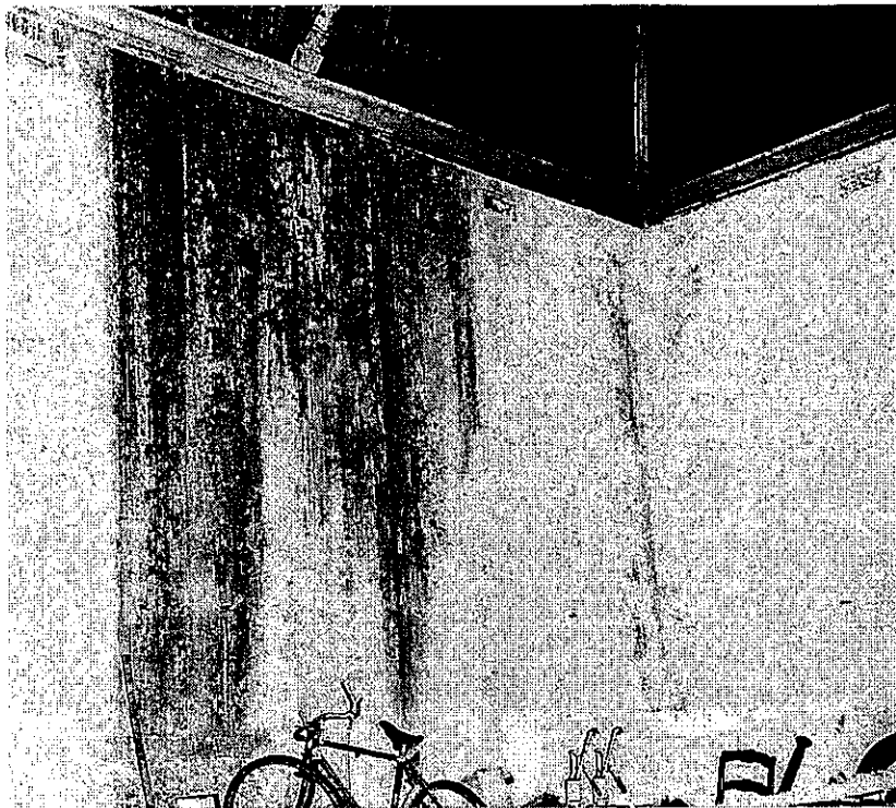
Figure 2.16: Interior detail of the Call Room, c.1974, showing evidence of substantial falling damp and deterioration in the coved timber ceiling. Source: City of Ballarat files.
