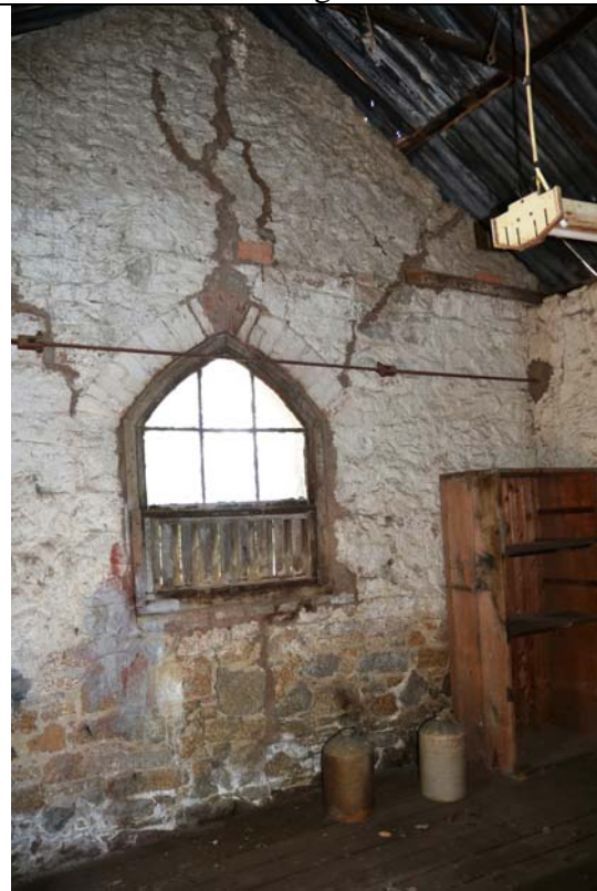
Photo 24 Interior of Tack Room (Room 1) looking west showing window with timber vent section below.
