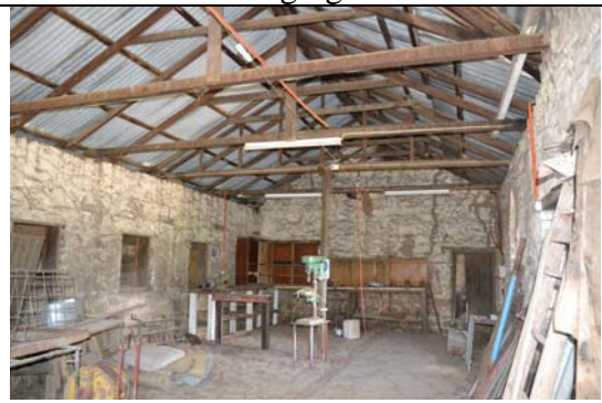
Photo 28 Stables (Room 3) looking south showing openings in east wall and door to Loose boxes (Room 4) in south wall.
