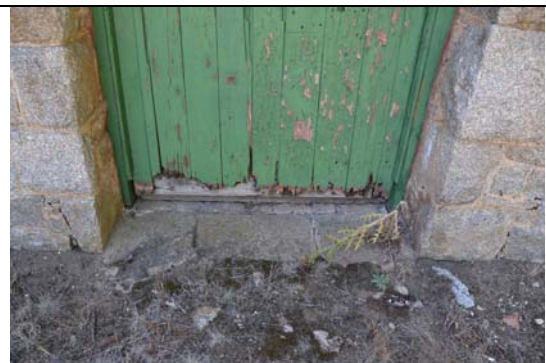
Photo 6 West wall door showing damage to base.
