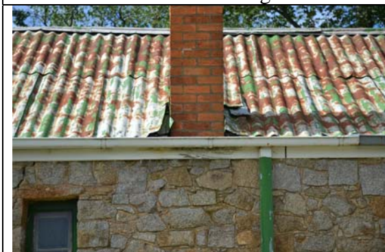
Photo 19 North wall, detail of chimney showing flashing problem.
