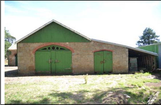
Photo 7 South face of stables showing doors to loose boxes and extension of skillion to form store area
