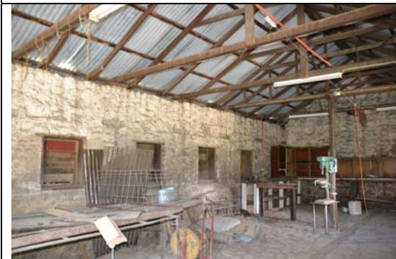
Photo 29 Stables (Room 3) looking south east showing openings in east wall
