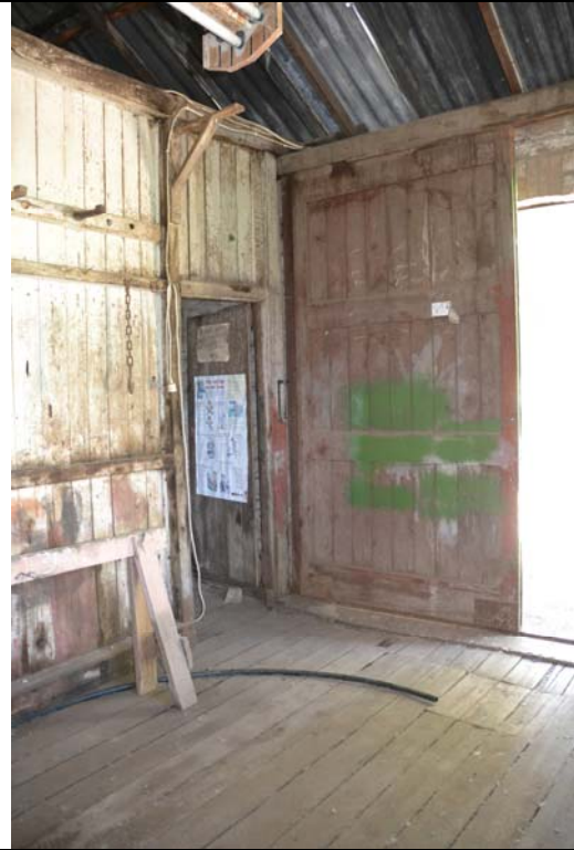
Photo 22 Interior of Tack Room (Room 1) looking south east showing timber partition wall on east, timber floor and external timber sliding door
