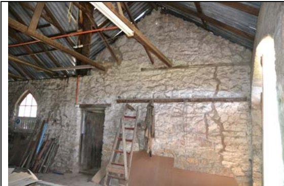
Photo 31 Stables (Room 3) looking west showing gable roof and internal stone wall of Groom's Room (Room 2)
