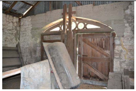
Photo 38 Loose Boxes (Room 4) Looking south to doorway showing introduced concrete in wall
