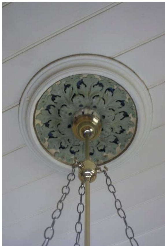
Figure 29. detail of ceiling rose and timber board ceiling in front parlour (Room 2)
