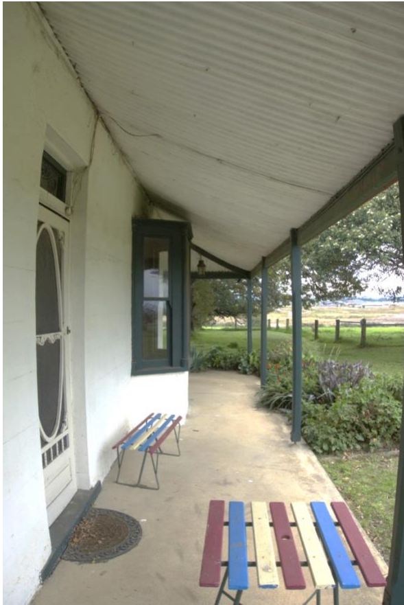
Figure 21. Detail of east (front) elevation showing convex, self-supporting verandah and bay window
