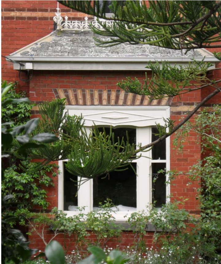
Figure 7. Detail of the front bay window. Note the timber cover to conceal external roller blinds. (source: Context 2016)
