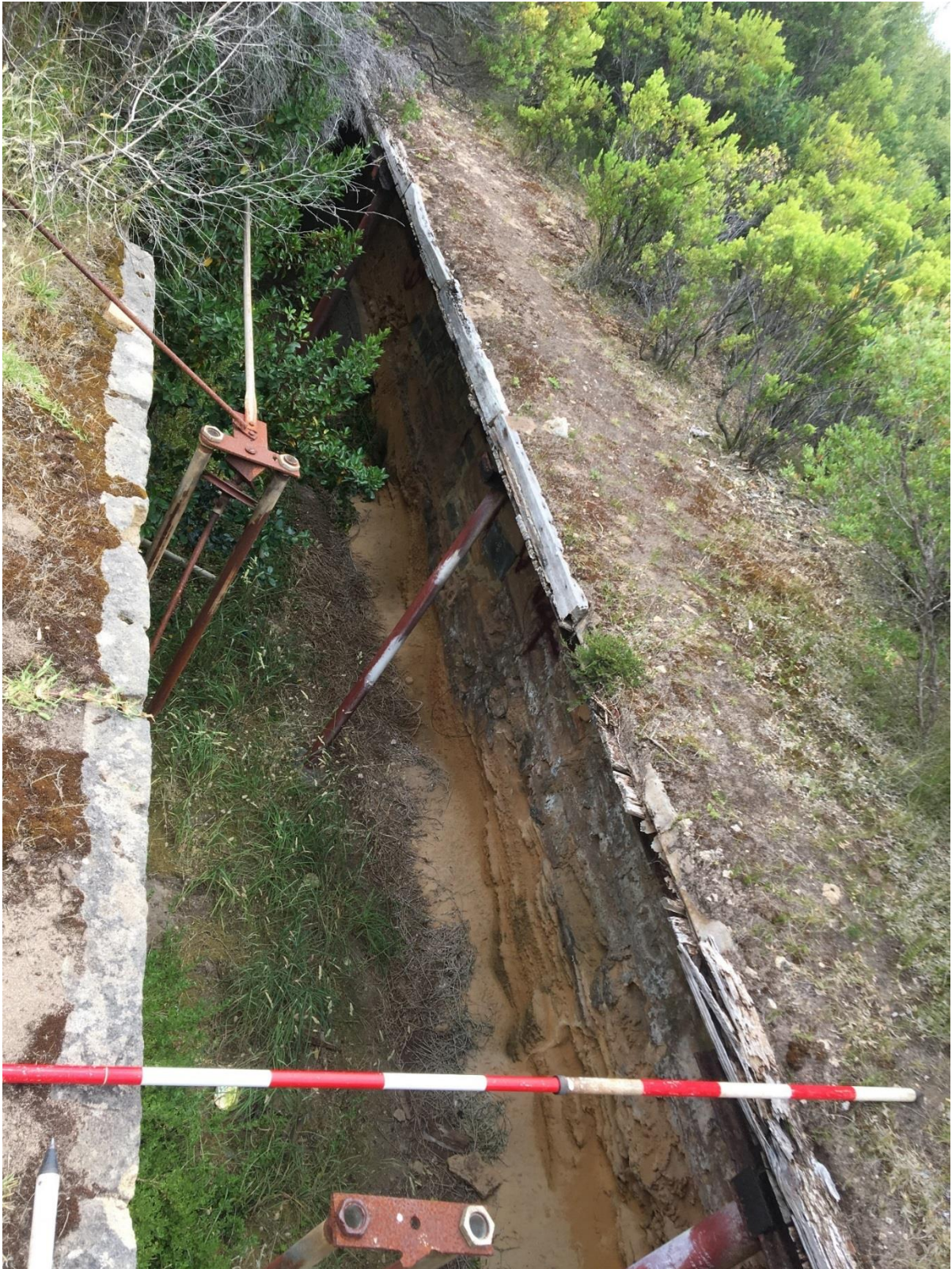
Figure 11 Constructed trench at forward (northern) face of rifle butts. Timbre and masonry construction material visible as well as steel components of target frames.
