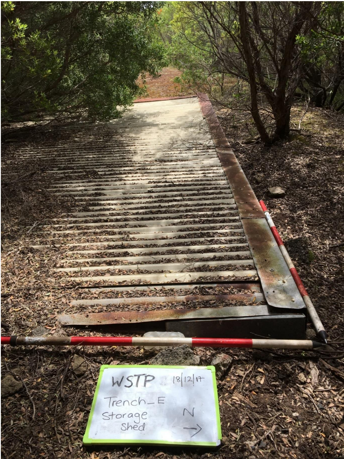
Figure 13 Roofed eastern extent of trench, identified as a storage area. The roofing of the sub-surface trench is at ground level and constructed from galvanized corrugated iron.
