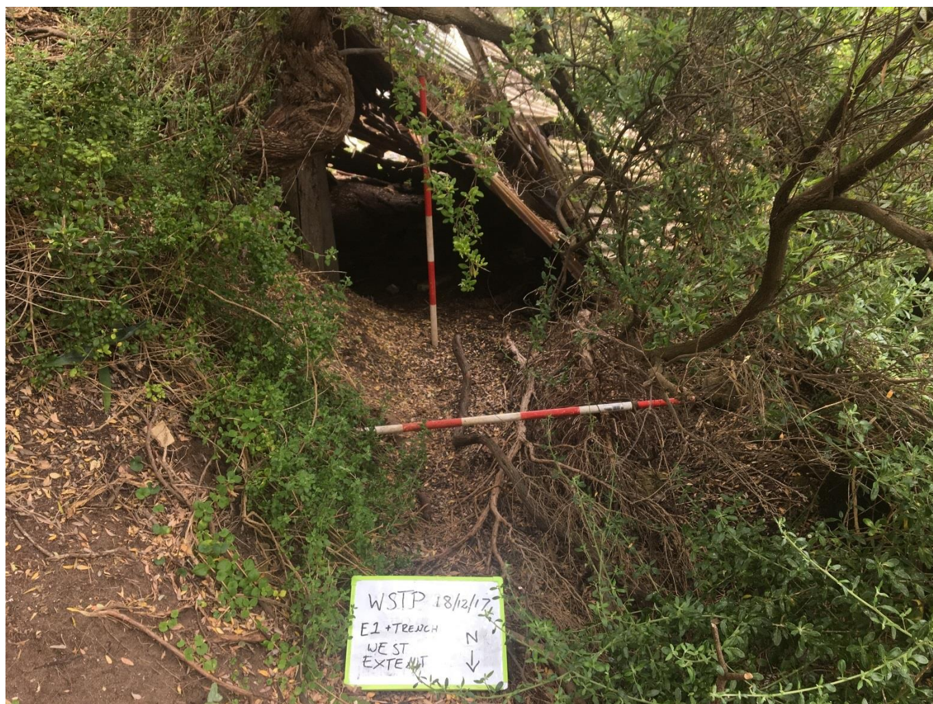
Figure 3: Western extent of the trench, showing collapsed roofing of corrugated iron sheeting. Facing east.
