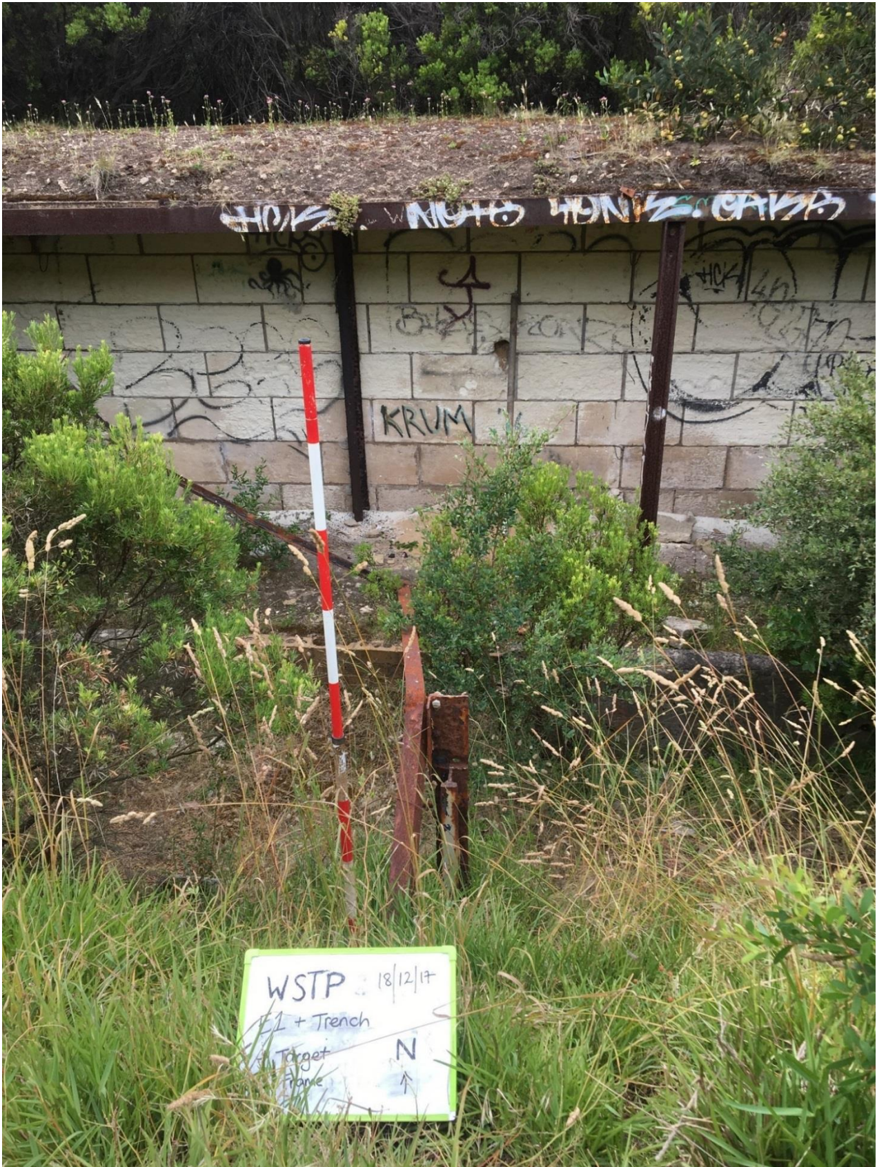
Figure 14 Recent components of trench at eastern extent. Materials used include masonry, and iron components, including supports made from reused rail track
