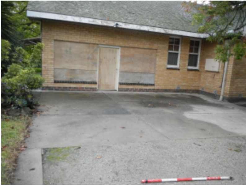
Centre of the site facing east across concrete paved area towards extant dwelling
