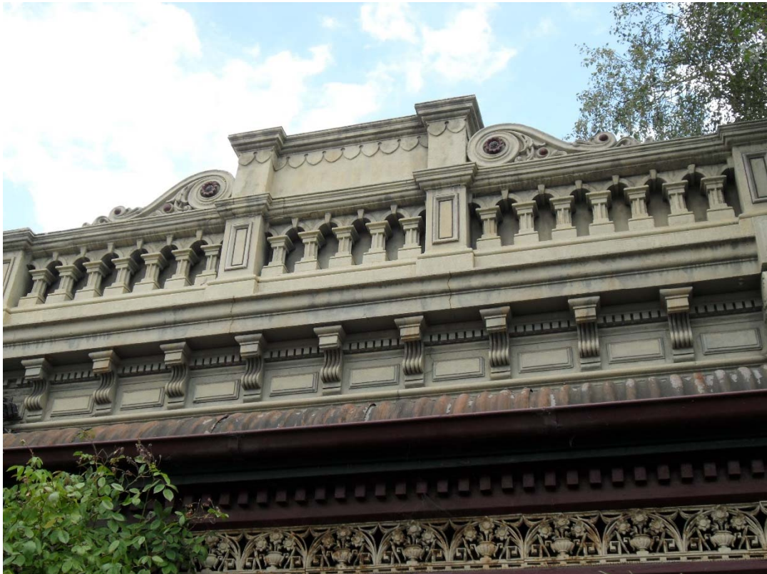
Figure 2. Detail of the verandah roof and parapet of 64 High Street (source: Context 2016)
