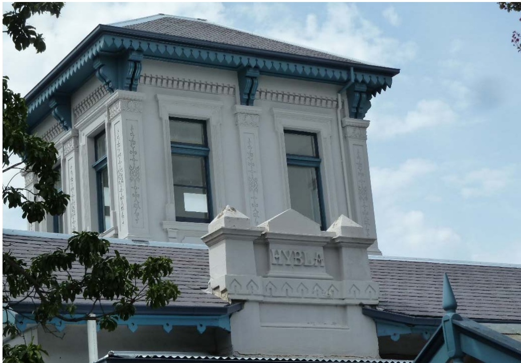
Figure 7. Detail of landmark tower and unusual name plate projecting above the main roof of the building. (source: Context 2016)
