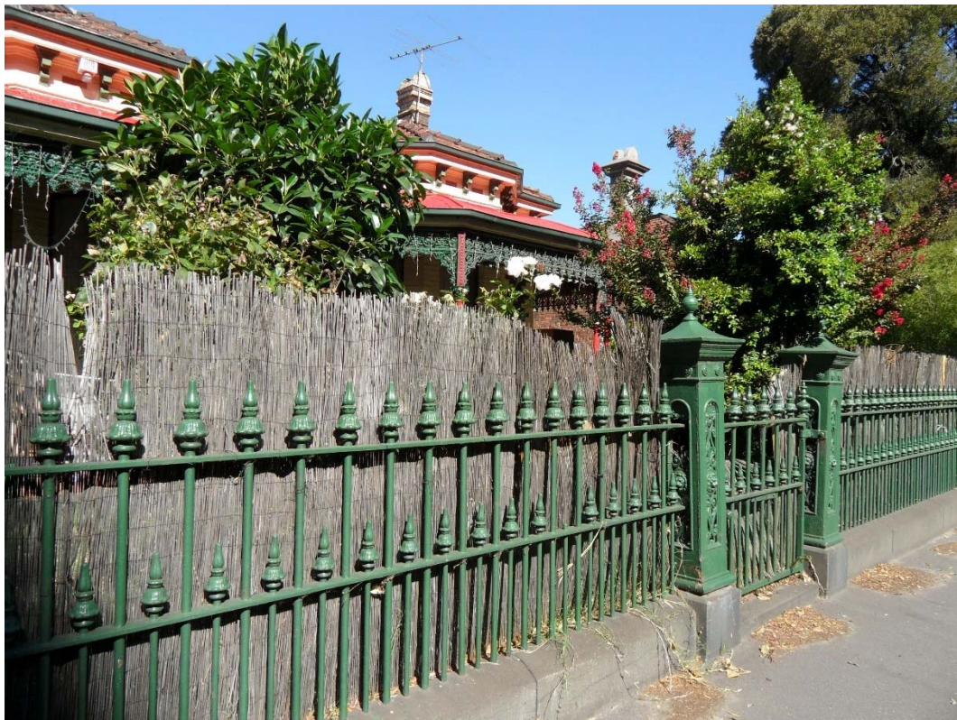
Figure 7. Detail of intact iron palisade fence with decorative posts and gate (source: Context 2016).
