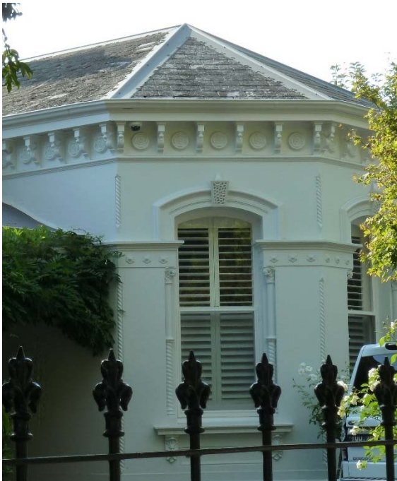
Figure 3. Detail of front projecting canted bay with fine cast and run detailing to bay windows (source: Context 2016)
