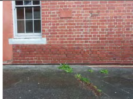
Photo 3.48: Former School (Building 4), detail of deteriorated pointing in brickwork.
