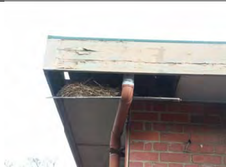
Photo 3.50: Former School (Building 4): detail of damaged eaves (south-east corner) with bird's nest.
