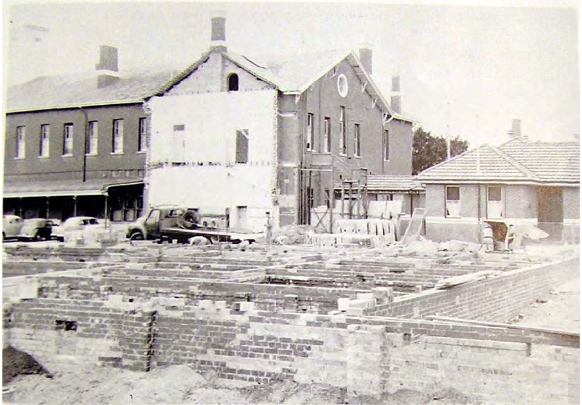
Figure 2.15: Demolition in progress of the east wing of the old orphanage building, 1959. Source: Annual Report, 1959.
