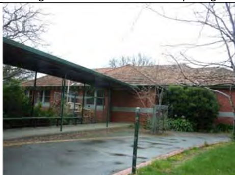
Photo 3.27: Former Toddlers' Block (Building 1), west elevation showing bricked up doorway and introduced walkway shelter.
