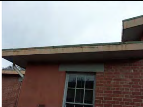
Photo 3.49: Former School (Building 4), detail of deteriorated eaves fascia.
