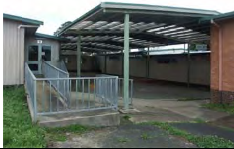
Photo 3.79: Former Bluebird's Cottage (Building 9) showing introduced portal frame provided an open covered area east of the brick building.
