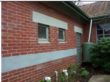
Photo 3.25: Former Toddlers' Block (Building 1), detail of north wall within courtyard showing altered window and door openings.
