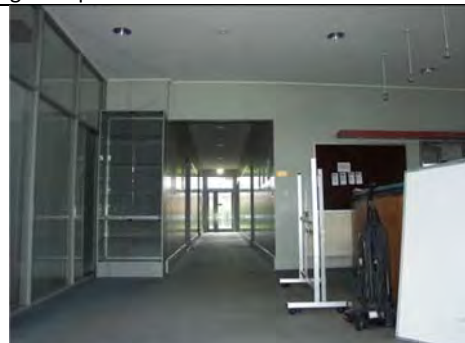
Photo 3.28: Former Toddlers' Block (Building 1), interior from front entrance looking south along corridor.
