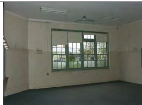
Photo 3.52: Former School (Building 4), interior of front classroom with original corner fireplace (now blocked up).
