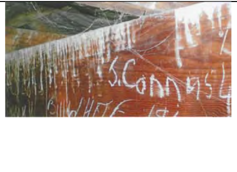
Photo 3.70b: Former Gymnasium (1907 construction), detail of roof beam with writing of former residents and dates. Source: City of Ballarat.
