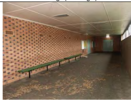
Photo 3.68: Covered way of the north wing of the former Service Block, Dining Room & Intermediate Cottage (Building 9).
