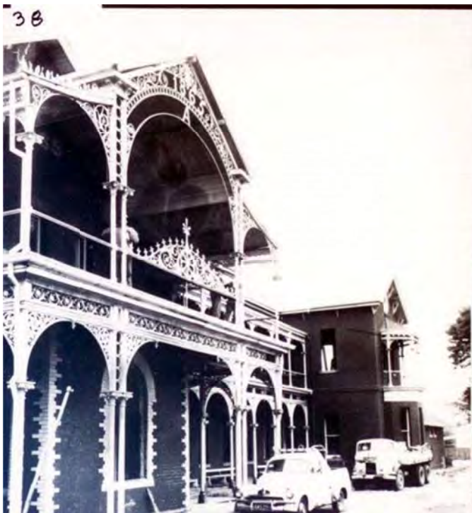
Figure 2.16: Demolition in progress of the front portion of the old orphanage building, 1965. Source: Central Highlands Regional Library, Ballarat, photo 38.
