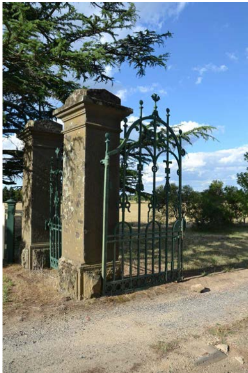
Photo 5 Pillar showing slight damage and rotation.
