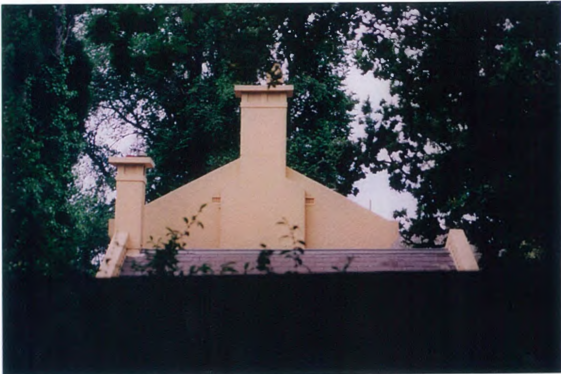
View from Albany Road showing Butler chimney design, and gable parapet, 1920 single storey extension in foreground
