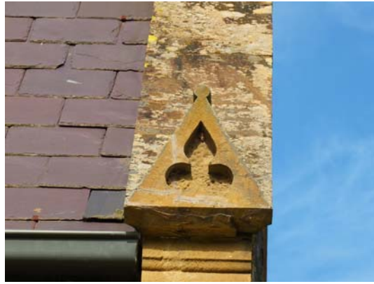
Detail of incised stylised trefoil motif in the end of a corbelling parapet cap.
