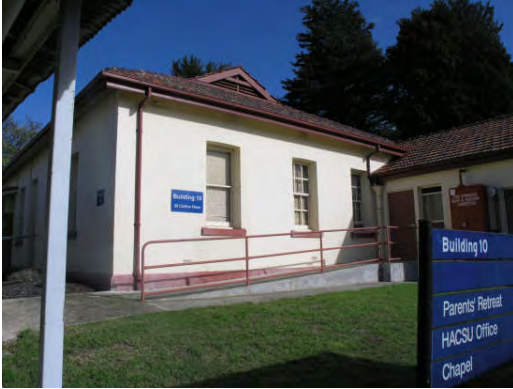
Photograph 7: North east elevation of B1 showing the extension to the right hand side of the original cottage Source: HLCD, 22.05.07
