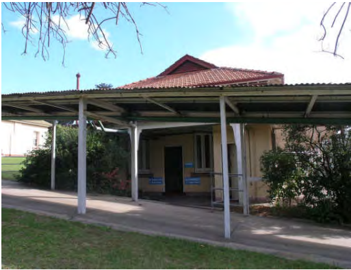
Photograph 25: South east elevation of B6 looking towards toilet block additions with concrete section of verandah floor Source: HLCD, 22.05.07
