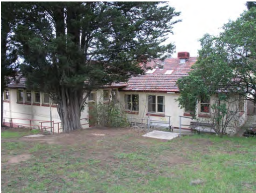
Photograph 6: North western elevation of B1 showing extension to original roofline Source: HLCD, 22.05.07
