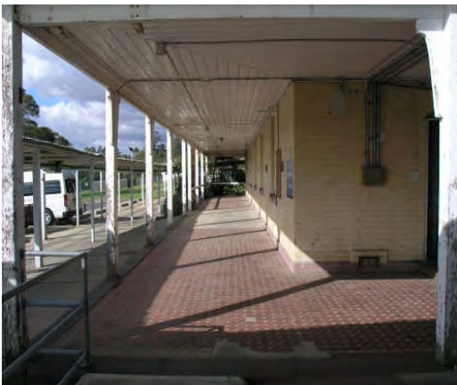
Photograph 26: Verandah along north eastern side of B6 showing concrete infill section Source: HLCD, 22.05.07
