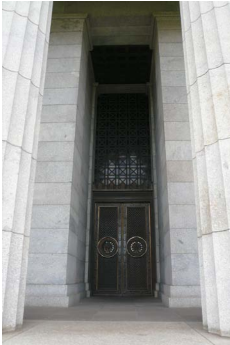
Figure 37 View of one of the doorway openings. This doorway is located within the entry portico to the south facing elevation.
