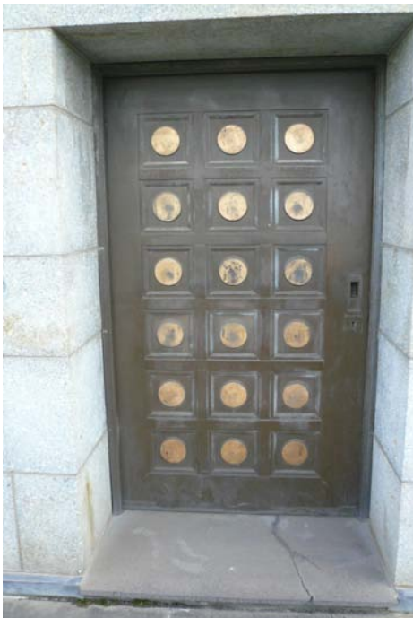
Figure 71 View of an original bronze sliding door. Note that this door is located on the east elevation to the lower balcony.
