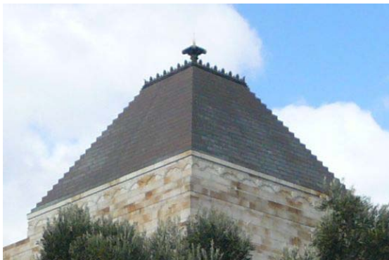
Figure 46 View of the northern and western slopes of the pyramidal main roof of the Shrine.
