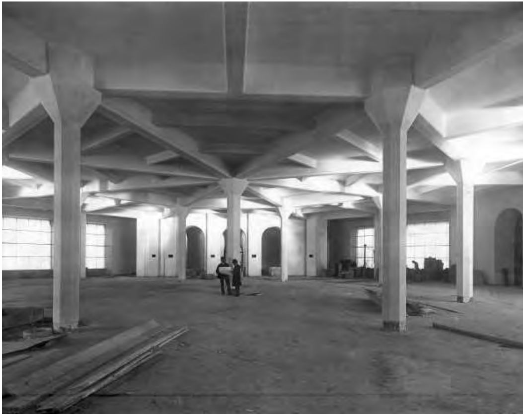
Figure 13 Interior of the ground floor Newspaper Room, below the new Reading Room, during its construction, c. 1913.
