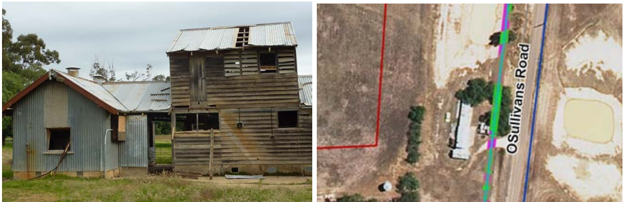
Left: East elevation of the former store (left) and the former seed extraction room (right). Right: Aerial view, 2010 (Source: City of Greater Bendigo).
