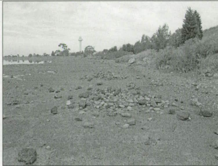
Straight section of Limeburners Point Causeway leading to Lime Kilns. Note sporadic clusters of roadway materials.
