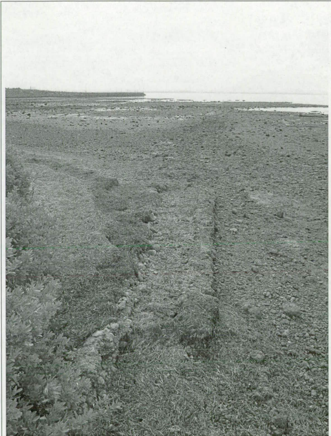
Intact section of the Limeburners Point Causeway located at the end of the curved section above the high water mark (facing north)
