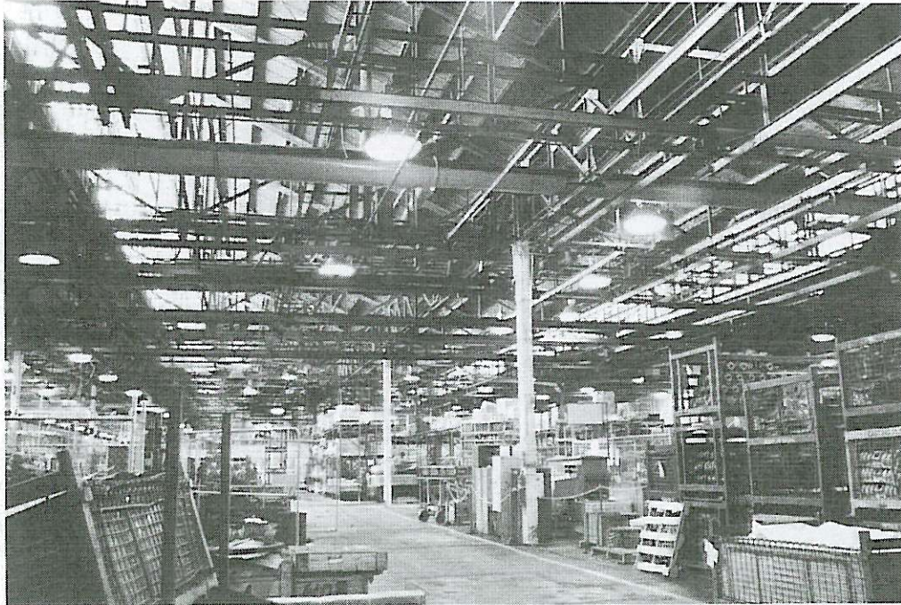
Ford Motor Company Building, North Geelong. Interior view of roof truss systems.
