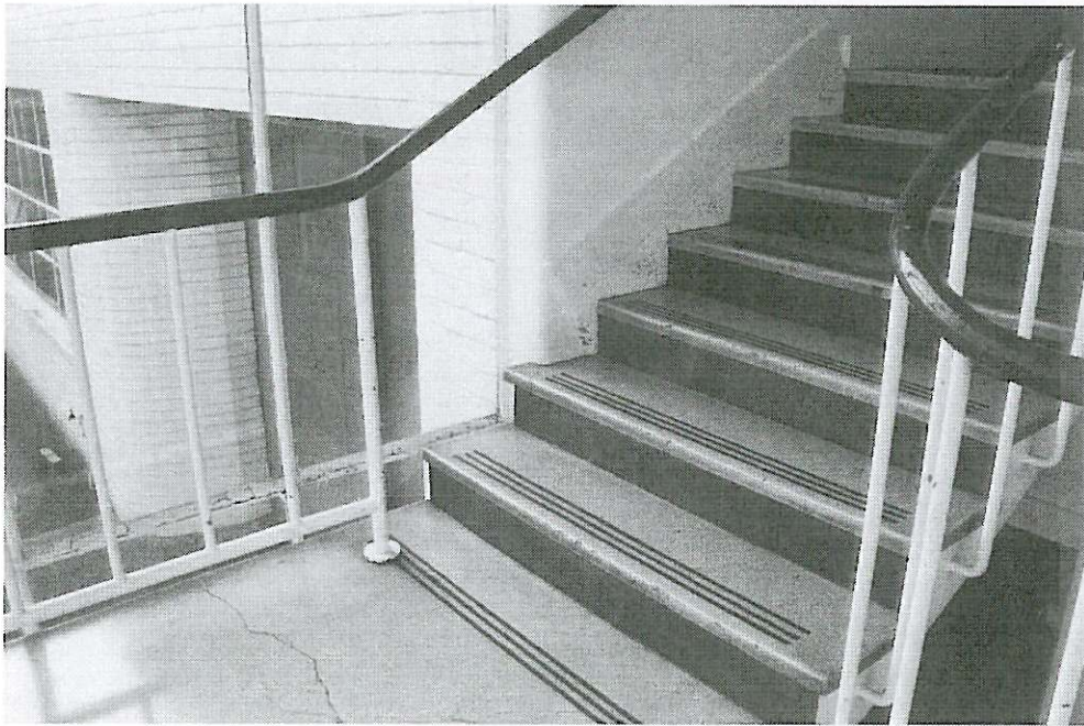
Stair detail. Note the blue tiled skirting has been over painted in white. The curved brick reveals and deep horizontal mortar joints are visible in this photograph.
