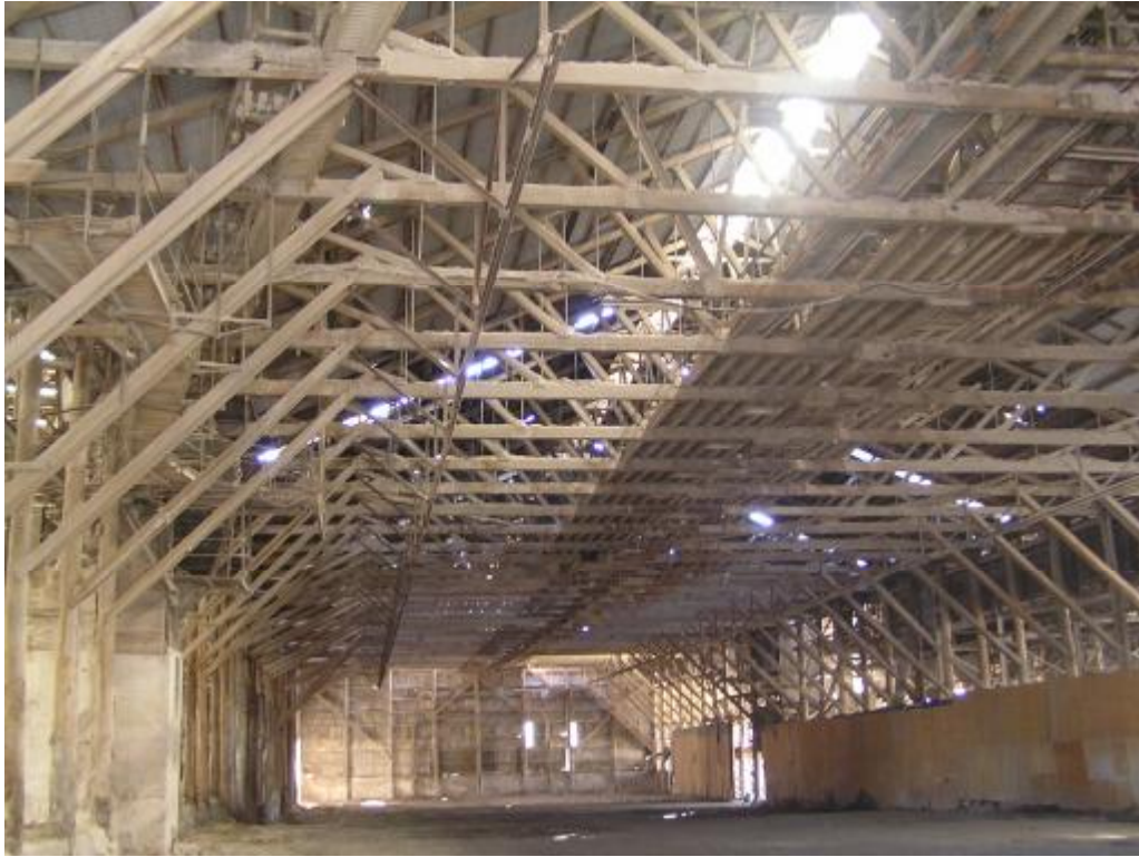
Figure 1 Interior of Shed 4 and 5, prior to demolition. Several of the poles and oregon beams and rafters have been retained for potential reuse in the interpretation scheme.
