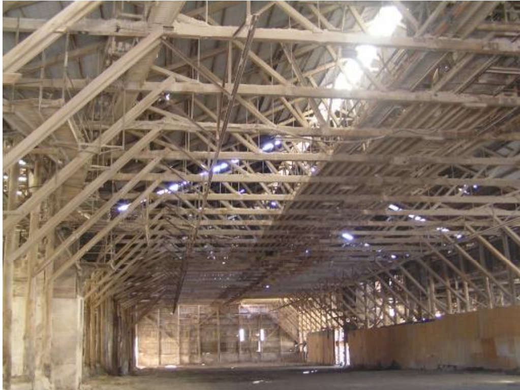
Figure 26 Interior of sheds 4, 5 & 6. Several of the poles and Oregon beams and rafters have been reused in the site interpretation.
