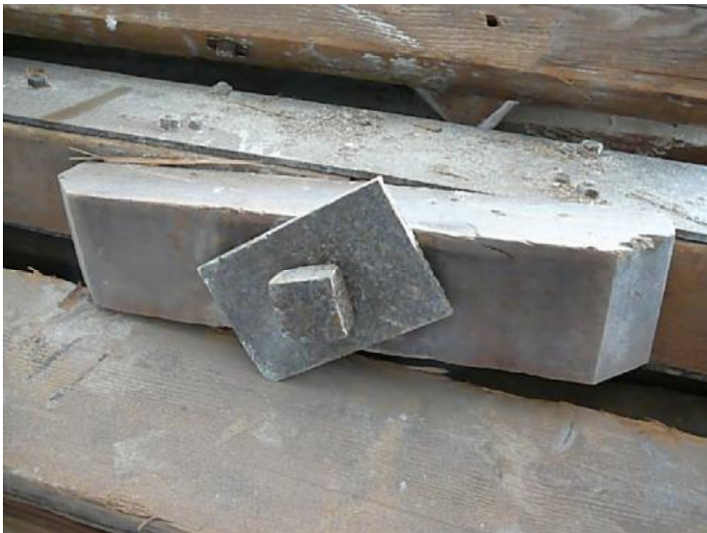
Figure 4 Example of tie bolt and washer plate with timber corbel affixed to one of the rafters.
