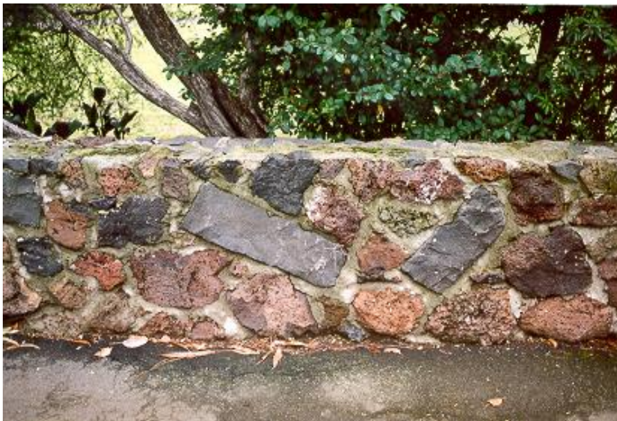
Fig 38 Extant stone wall to Yarraville Gardens along Hyde Street (reconstructed c.1966), shows poor workmanship in placement of stone and construction technique (wide mortar joints, vertical profile in mortared wall technique) (photograph Jill Orr-Young, 2000)
